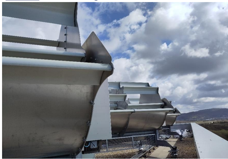
CISM Building 3x Crossflow wind turbines
